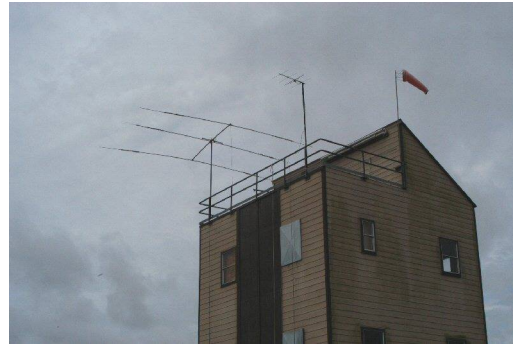
Antenna farm on building
